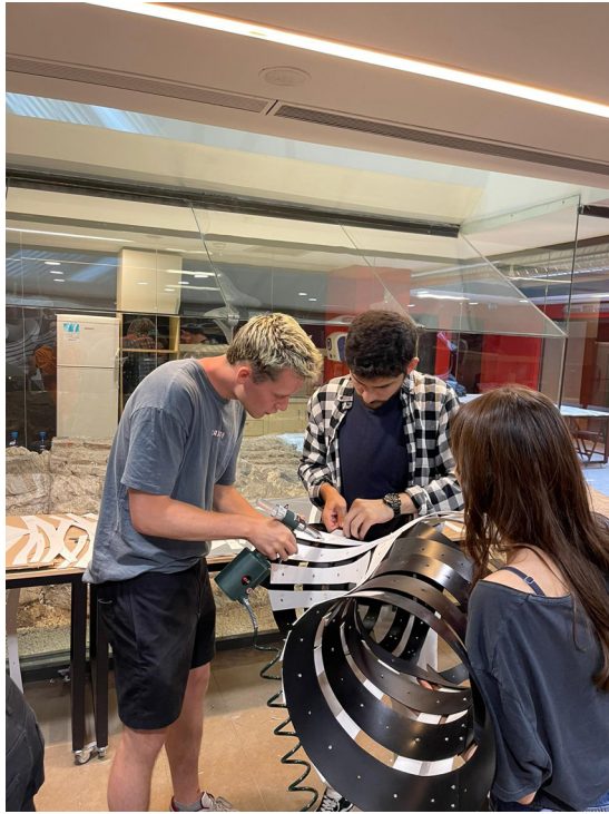
Figure 7: Construction of a part of the installation showing alignment and connection of black and white strips using rivet guns.
