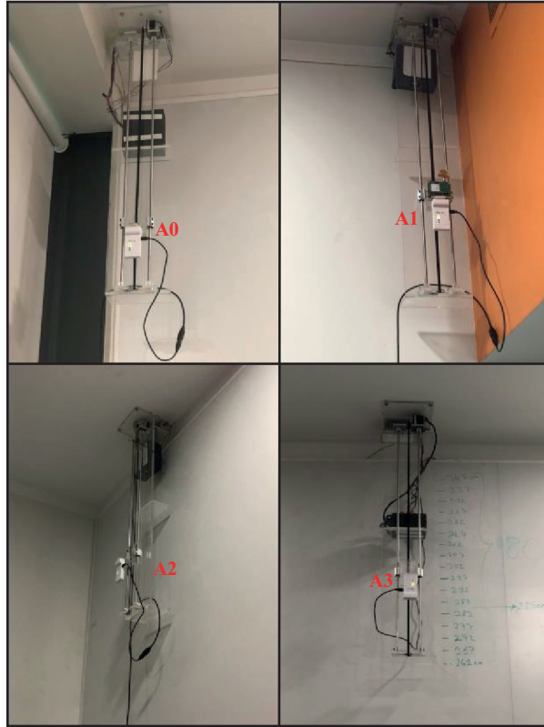
Figure 5. Adaptive ceiling system; four Decawave MDEK1001 UWB sensors (anchors) are mentioned as A0, A1, A2 and A3.
