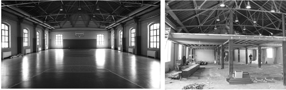
Figure 1. The spatial transformation that took in place in 2010. Note the second floor installed and wall divisions made for studios in right.
